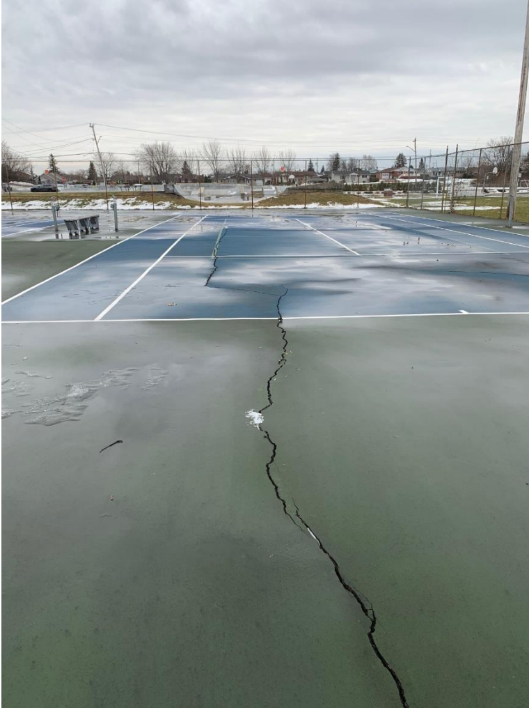
The picture shown above demonstrates an additional crack to the surface of the existing tennis court, forming in another direction from the first photo.
