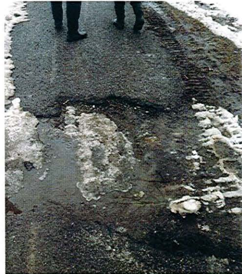
Figure 5: Existing asphalt pathway in disrepair
