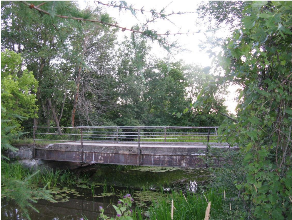
Picture 1. West Elevation. Note noticeable sag of the bridge. The corner at the left now supported by channel bolted to abutment.
