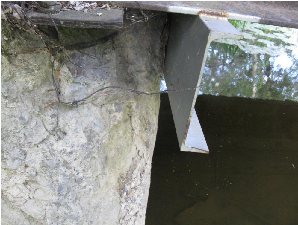
Picture 7. The northwest corner where bearing seat was lost and the end of girder is supported by channel. The other three corners have still residual bearing capacity.
