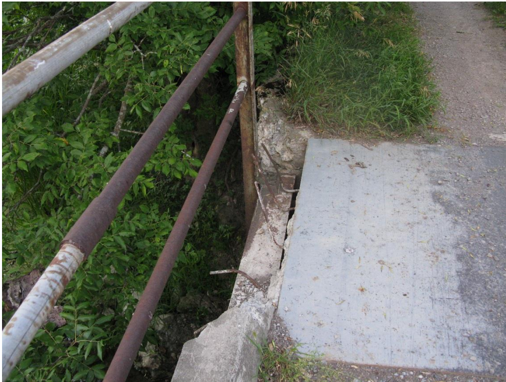
Picture 3. Curb and deck broken off at northwest corner and steel plate was installed.
