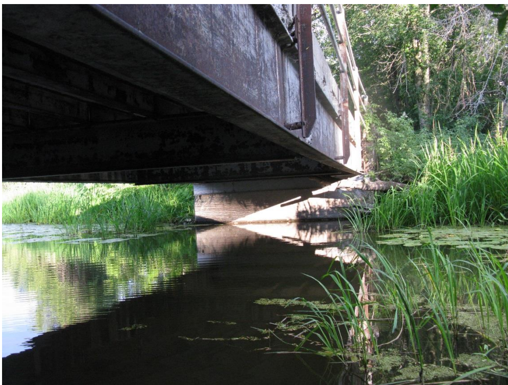
Picture 8. Overall view of underside. Note sag in girder.
