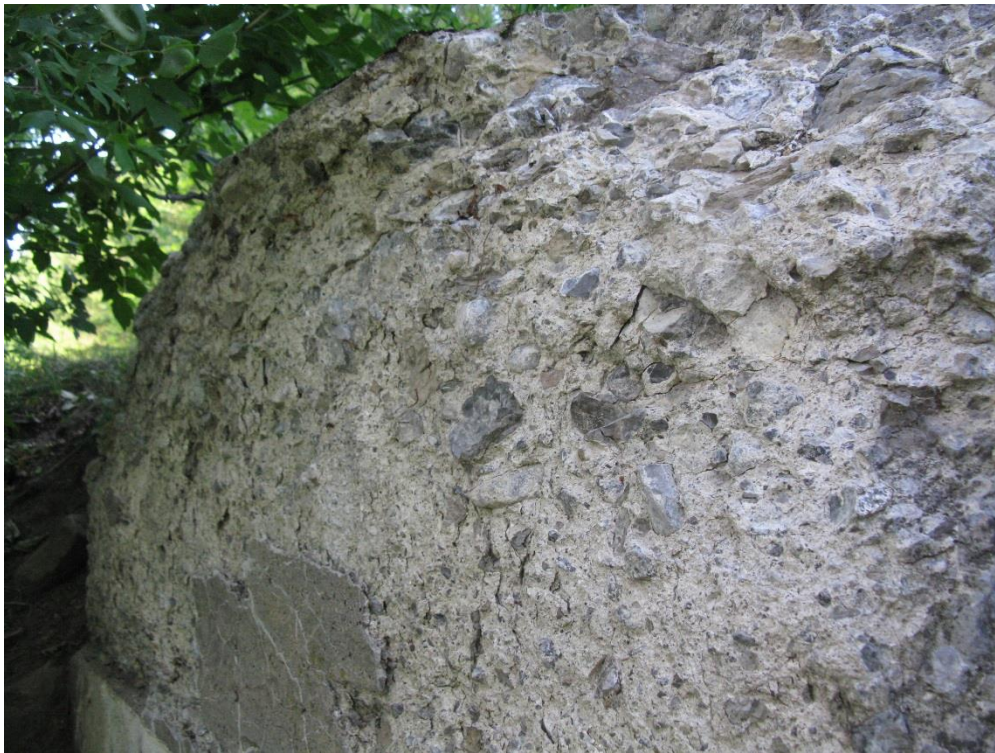
Picture 9. Disintegration of northwest wingwall.
