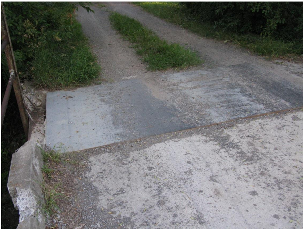
Picture 4. Heavy steel plate across the deck at the north end.
