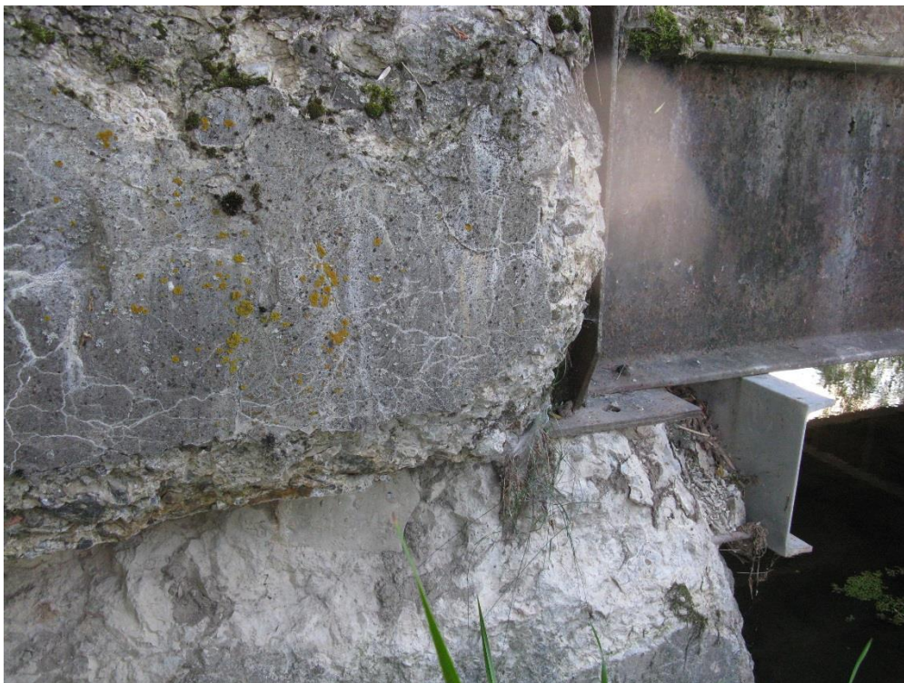
Picture 10. Disintegration of southeast wingwall.
