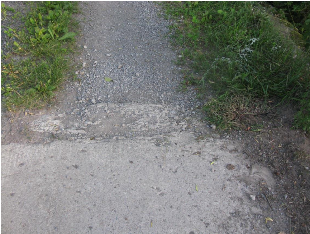
Picture 5. Completely disintegrating ballast walls in top of the road.
