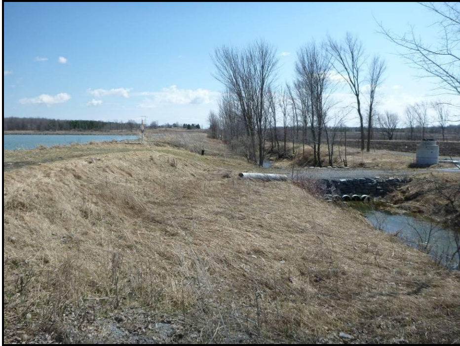
Image 11. Photograph of the dyke and extensive ditching along the western side of the study area, facing south. (PR15-08D014)
