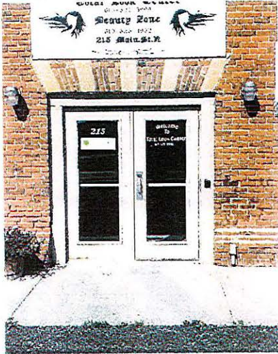
Replace with double door - no transom due to elaborate brick work.
